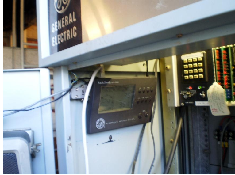
WX-200 Console Inside a Locked Radio Cabinet
